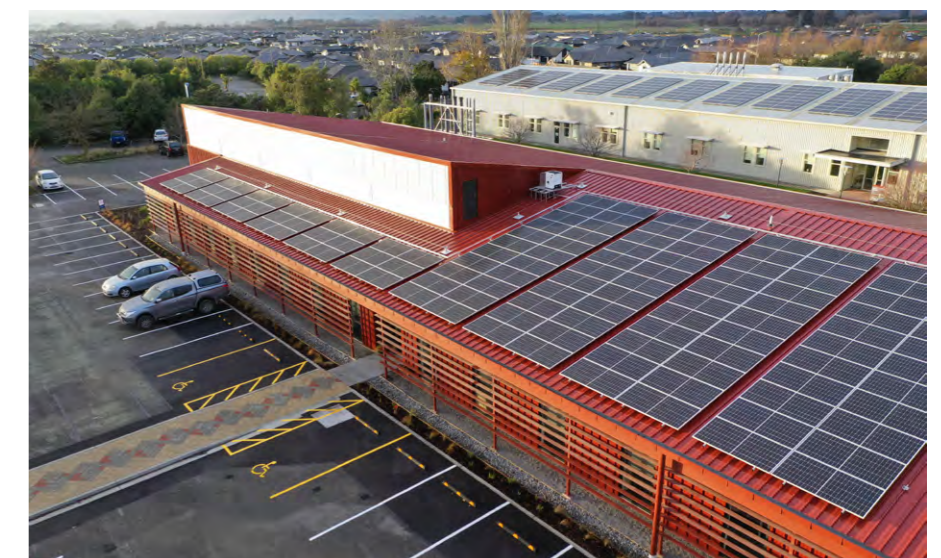
Solar array on the Agricultural Sciences Building contributing to our renewable energy generation.
