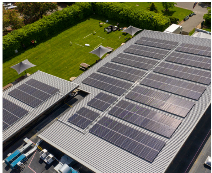
The first of the planned solar arrays on campus, Te Kete Ika solar array was completed in November 2019.
